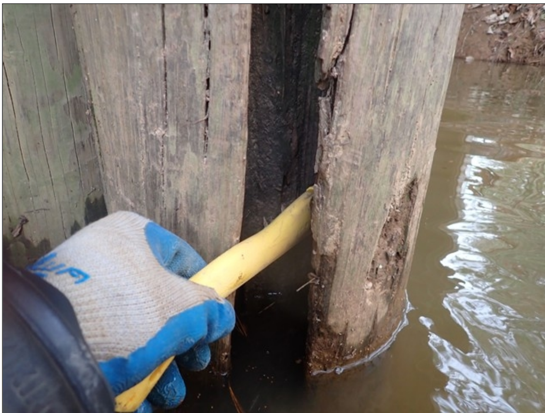
Bent 1 Pile 1: UNDERWATER INSPECTION: 3 FEET HIGH X 4 INCHES WIDE X 8 INCHES DEEP AREA OF DECAY FROM 1.5 FEET ABOVE WATERLINE TO 1.5 FEET BELOW WATERLINE. HELPER PILE IN PLACE.
