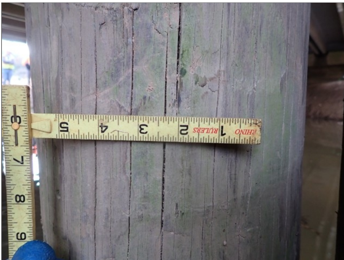
Bent 1 Pile 2: UNDERWATER INSPECTION: CHECKS TO 0.0312 INCH, SOFT TO 0.0312 INCH.
